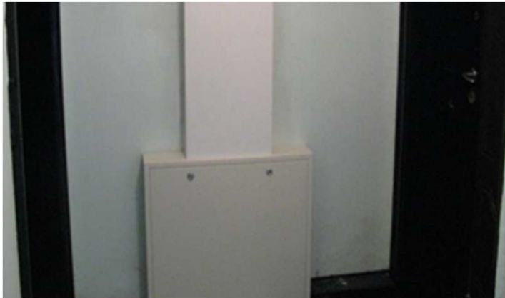
New heating installation located in common areas
