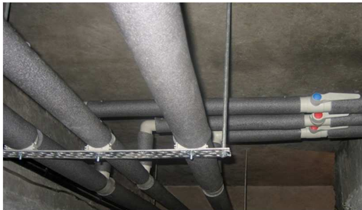
New domestic hot water installation (with insulation)
